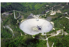
The failed cable was an auxiliary, anchored to the SE supporting tower. NAIC
